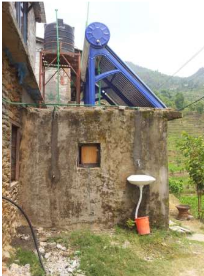
Picture 9: Basin and the hot water outlet
