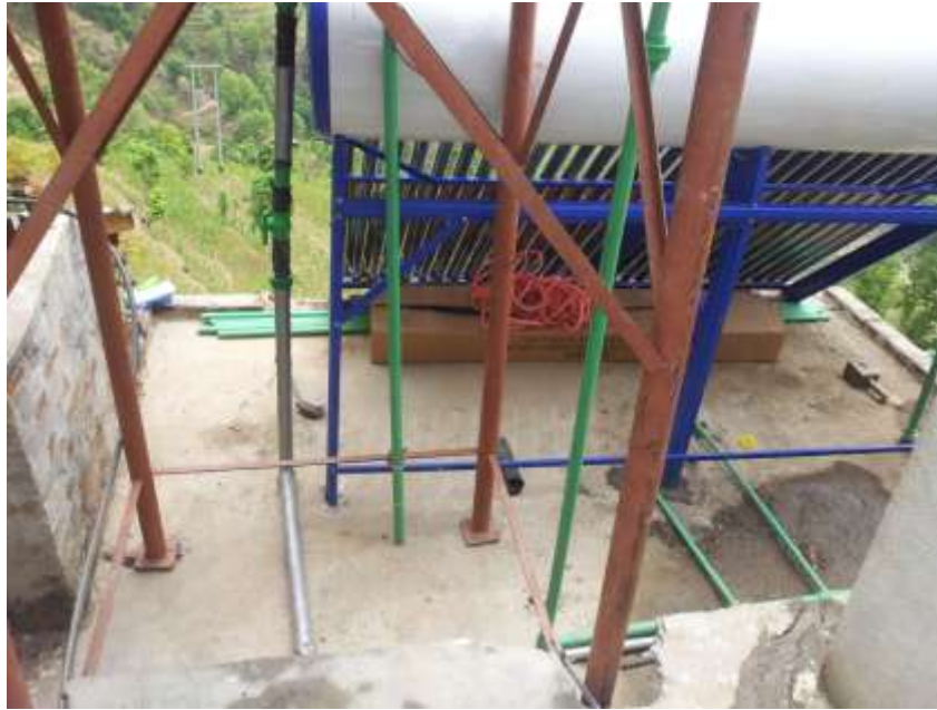
Picture 8: Piping network
