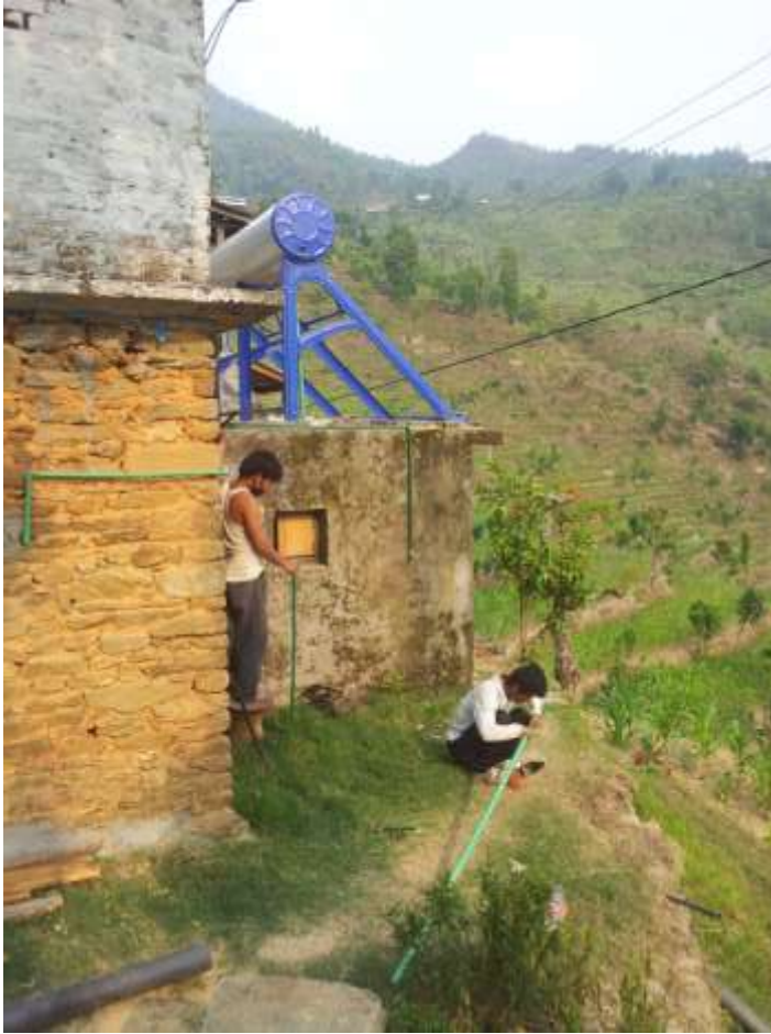
Picture 4 External outlets for hot and cold water
