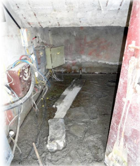
Water logging inside building
