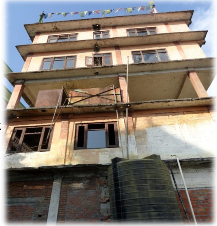
Unfinished exterior, broken windows & door, absence of floor slab in 1 st floor
