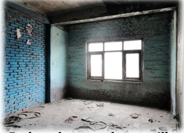
Broken plaster works, no grills
