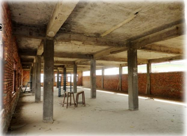
No proper planning of floors
